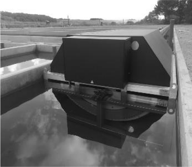
Effluent filtration from Danish troutfarm with HEX Drumfilter
